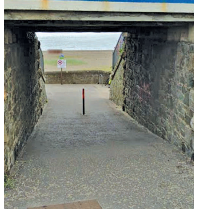
The Greystones South Beach archway, which has been prone to flooding
